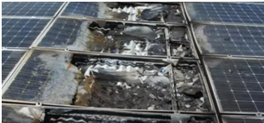
Fig. 2 Picture of a photovoltaic system D C series arc fault and fire damage
