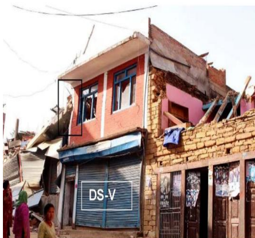
(A) Impact from a collapsing building
