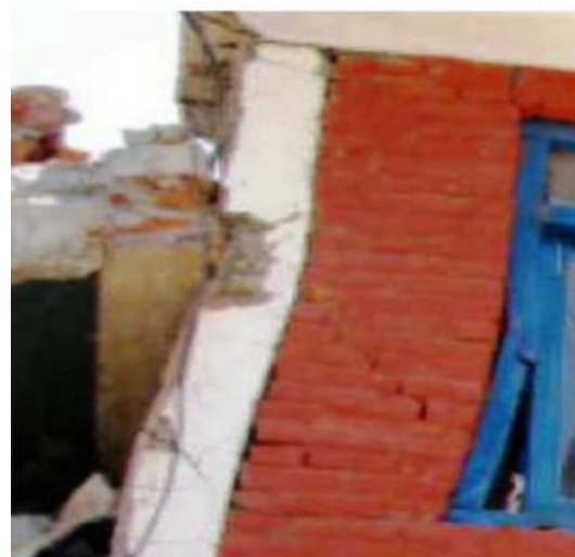
(B) Damage detail
